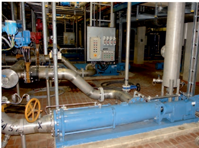
Feed pumps of the AE series for the filter beds
