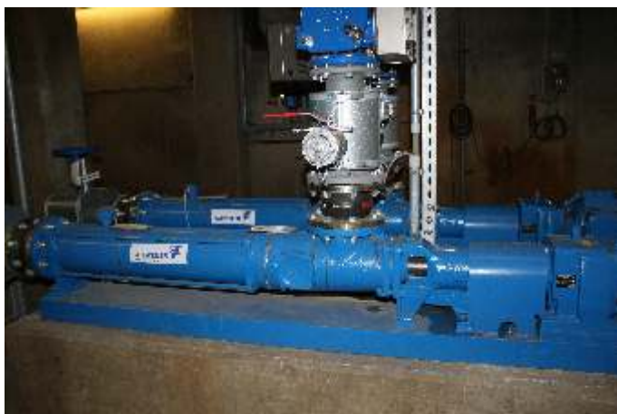
Approximately 80% of all pumps in the plant are from Allweiler®, including the thin sludge pumps in this photo.
