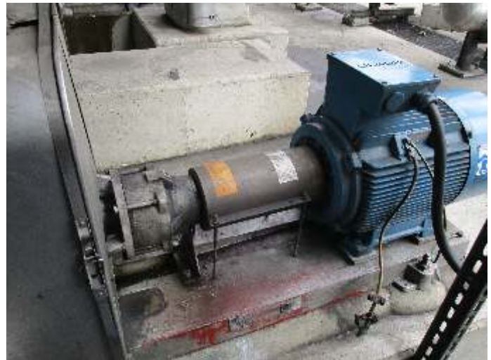
Centrifugal pump of the CTWH series providing column circulation (liquid: base oil)
