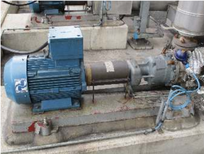
Magnetically-coupled centrifugal pump of the CNH-ML series providing column circulation (liquid: naphtha)
