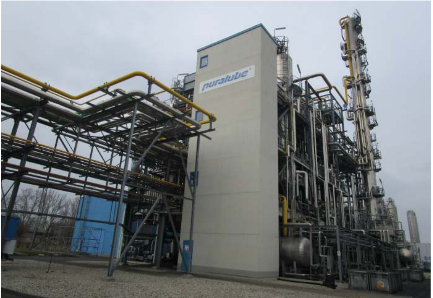
Process plant HyLube2
