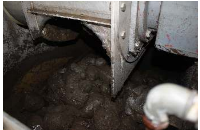
Sludge entering the pumping screws of the high-pressure pump.
