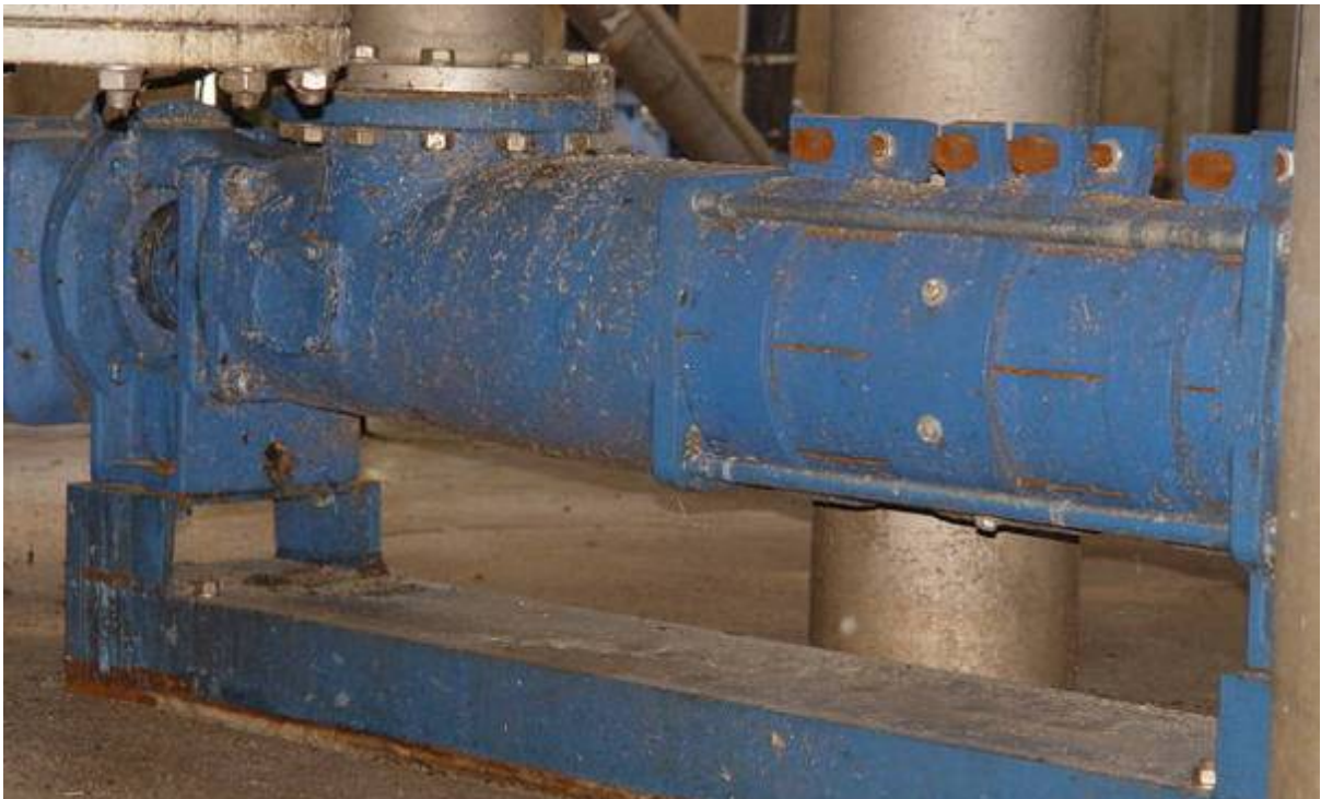
Allweiler progressing cavity pump of the AEB1E2700 series with readjustable stator; medium: biomass; capacity: 100 m 3 /hour; pressure: 2 bar.
