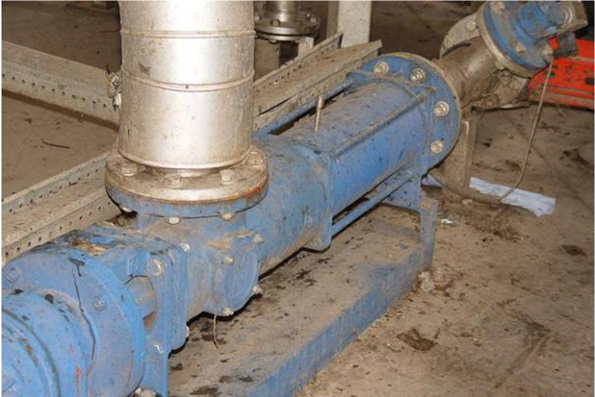
Allweiler progressing cavity pump of the AEB1E750 series; liquid: biomass at 75 °C; capacity: 18 m 3 /hour; pressure: 2 to 4 bar.
