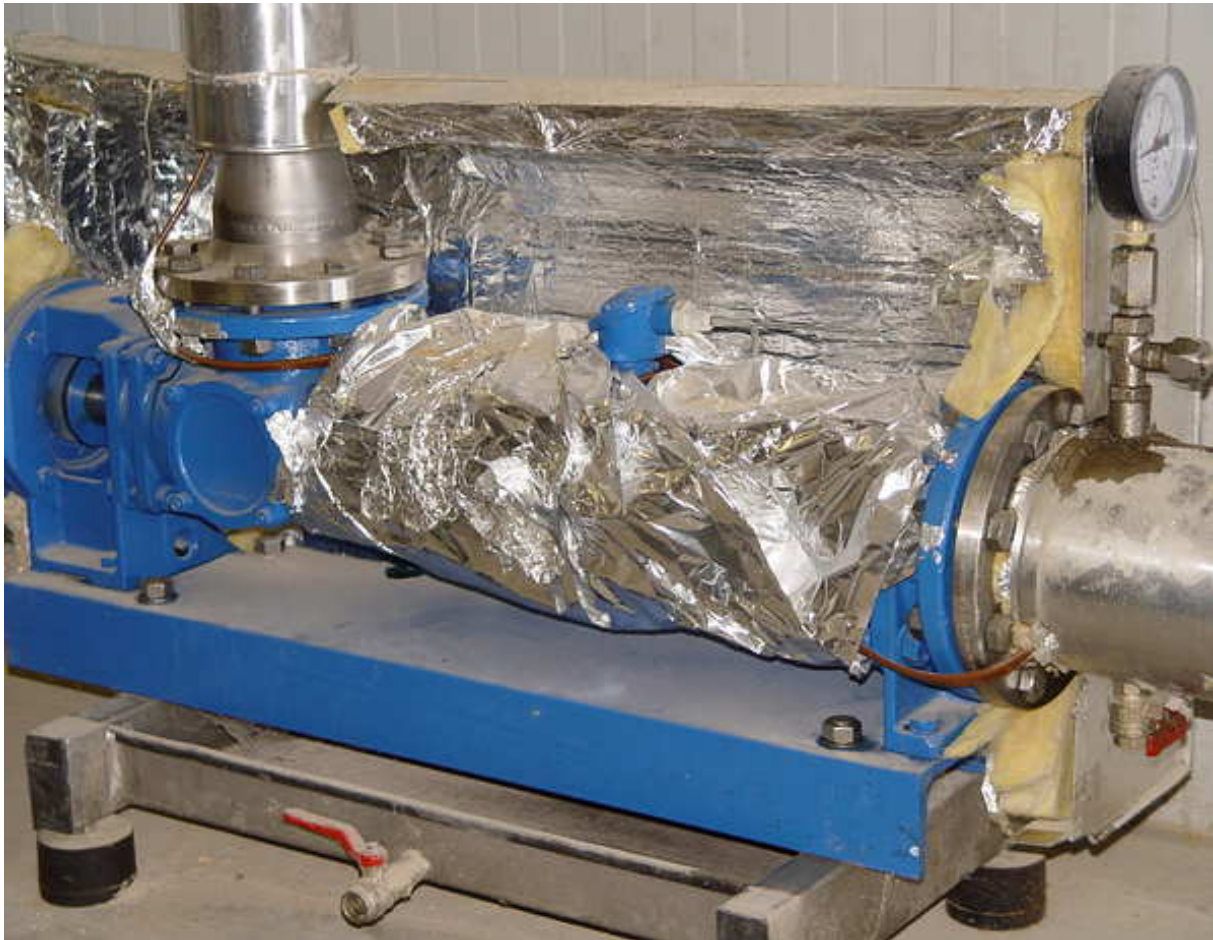
Allweiler progressing cavity pump of the AEB1E380 series; liquid: fat; volume 12,000 kg/h; pressure: 2 bar; temperature: 30-65 °C; distance: 65 m.
